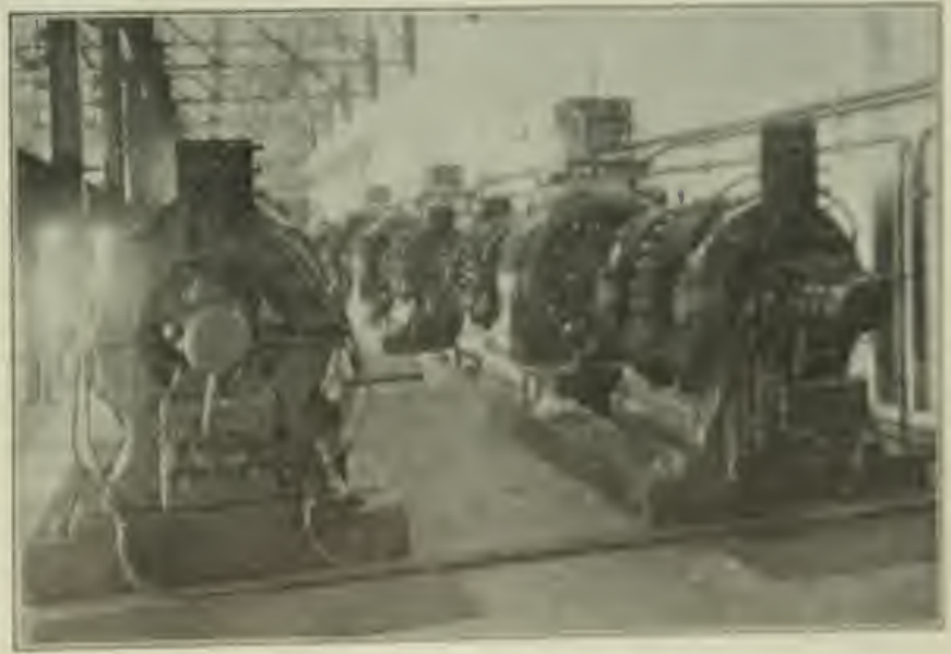
FIG. 12. TURBINE AND GENERATORS
